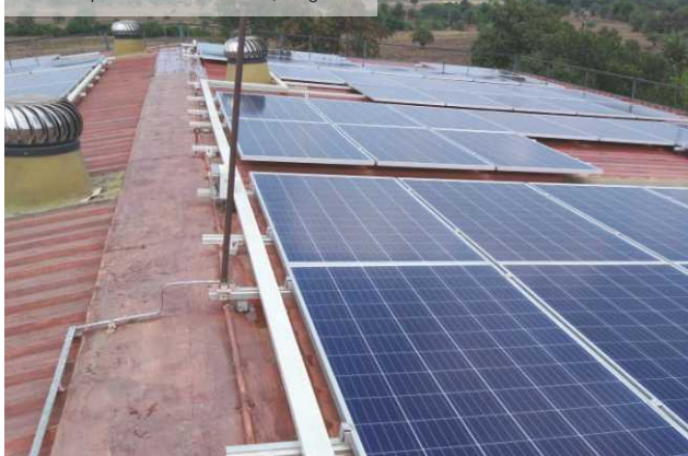
Rooftop Solar Panels –Unit 2, Palghar
